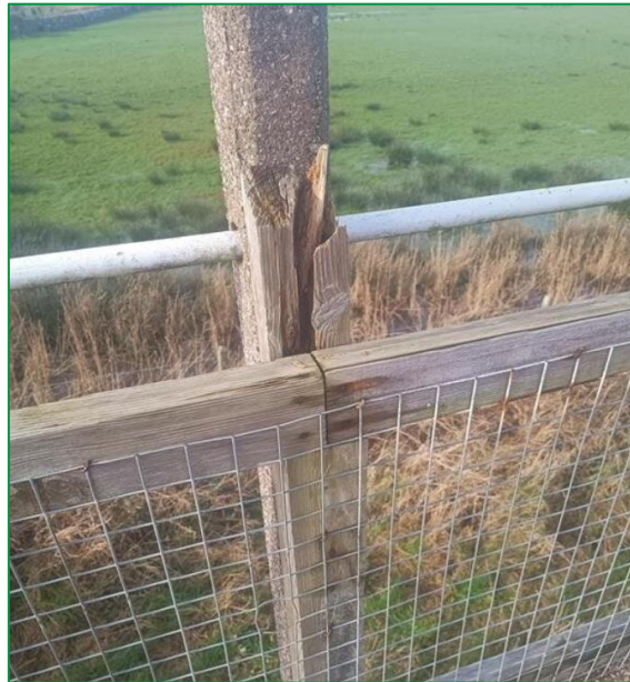
Esiampl o gyflwr y ffens presennol Example Image of current fence condition
